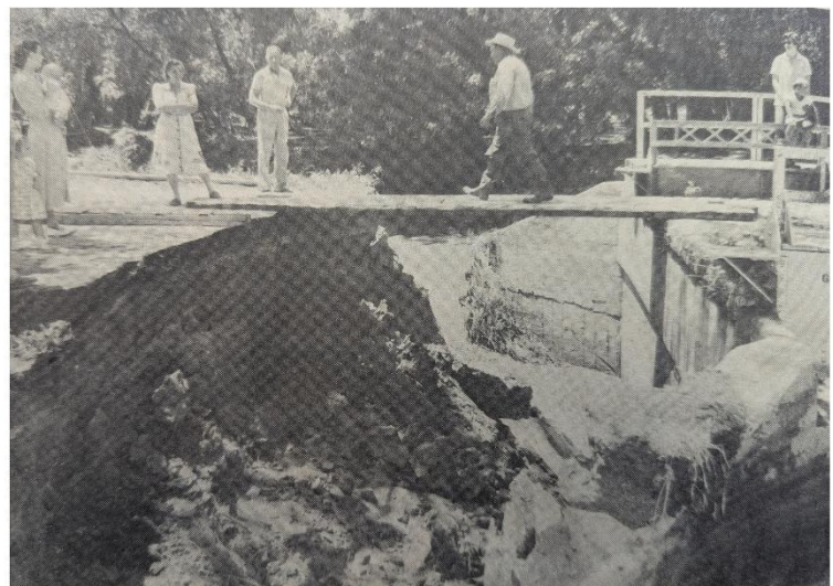
When water couldn't go under the bridge because of all the trees, it went around, cutting away soil at the bridge's east abutment. Bridge planks were placed over the cut to allow residents on the east side to cross over to the west side of town. (Photo courtesy of E.N. Berry, Jr.)
